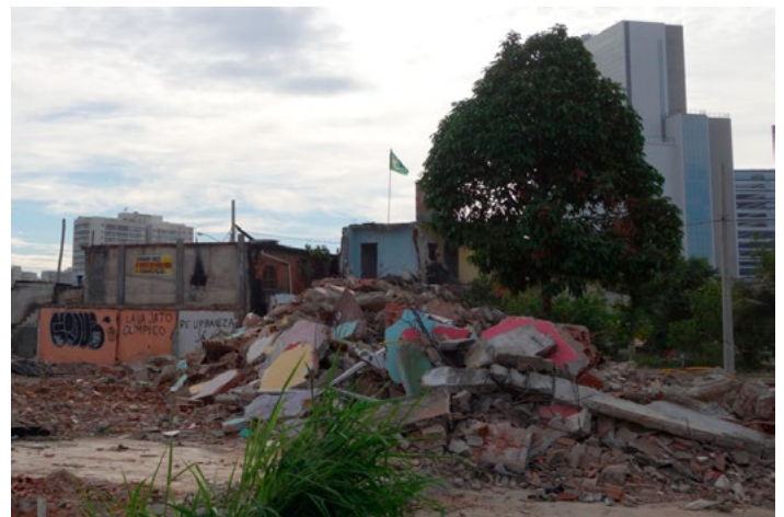
The remaining residents in Vila Autódromo live among the rubble of demolished houses while the Olympic Park rises in the background. The graffiti calls for the on-site upgrading of Vila Autódromo, and refers to the involvement of Olympic construction projects in the unfolding corruption scandal "Lava Jato".
